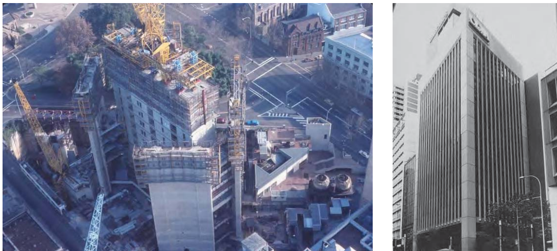
Figure 30 Second stage of the Qantas International Centre under construction, showing the relationship between the central core and the canted columns (left); former South British Insurance building in Hunter Street (right).
